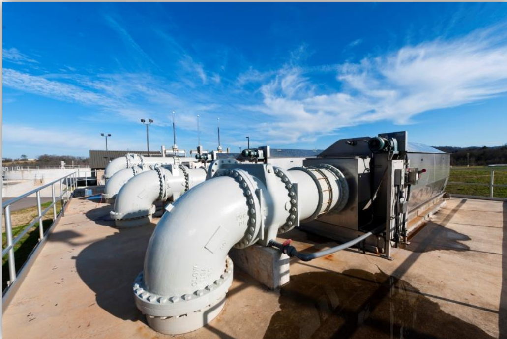
Internally Fed Rotary Drum Screens w/ 0.08-inch openings Maryville Regional Wastewater Treatment Plant Maryville, Tennessee
