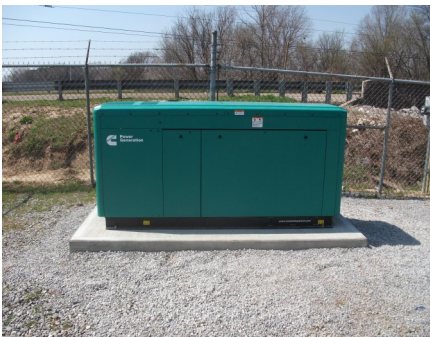
Pictured left is one of three CDBG funded Generators Halls, Tennessee
