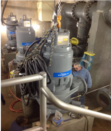
Pictured left is the installation of three 150 HP Flygt dry pit submersible pumps Janalee Drive Sewage Pumping Station Henderson, Kentucky
