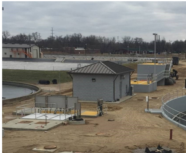
Pictured above is New Electrical Room and Diversion Structures North Wastewater Treatment Plant Henderson, Kentucky
